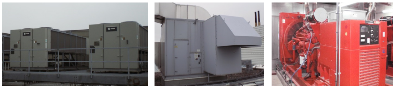
From Left: Reciprocating chillers, rooftop air handling unit, emergency generator set
